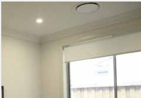
8. SAMSUNG 12KW DUCTED AIR CONDITIONING
